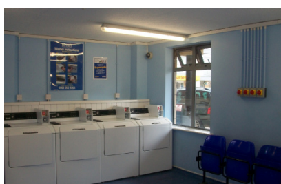
On-site laundry facilities
